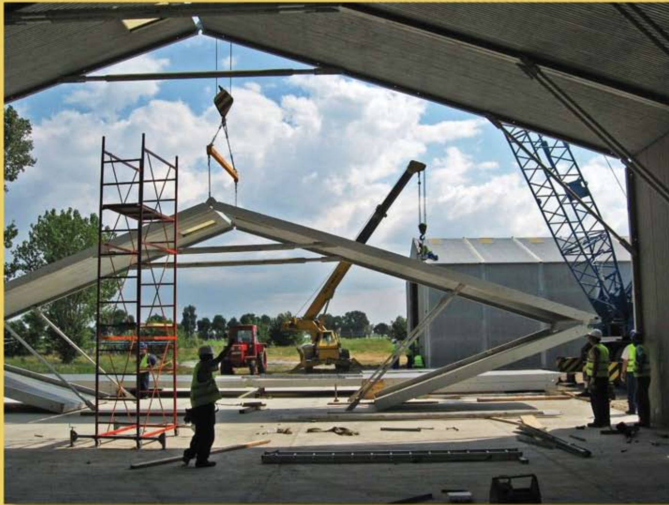
Contractors work to erect a building at the TFOS. (Photographs by SKE Group)
